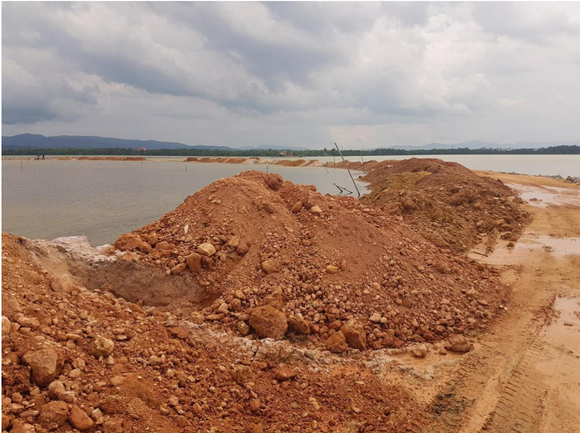
Figure 1 . Piles of lateric soil are dumped into the Kendari Bay as part of ongoing reclamation projects. This photo, from 2018, shows the early-stage construction of a parking lot over a kilometer offshore. Similar soils are washed into the bay as alluvial sediment, furthering rapid sedimentation in the bay (Source Author's own).
