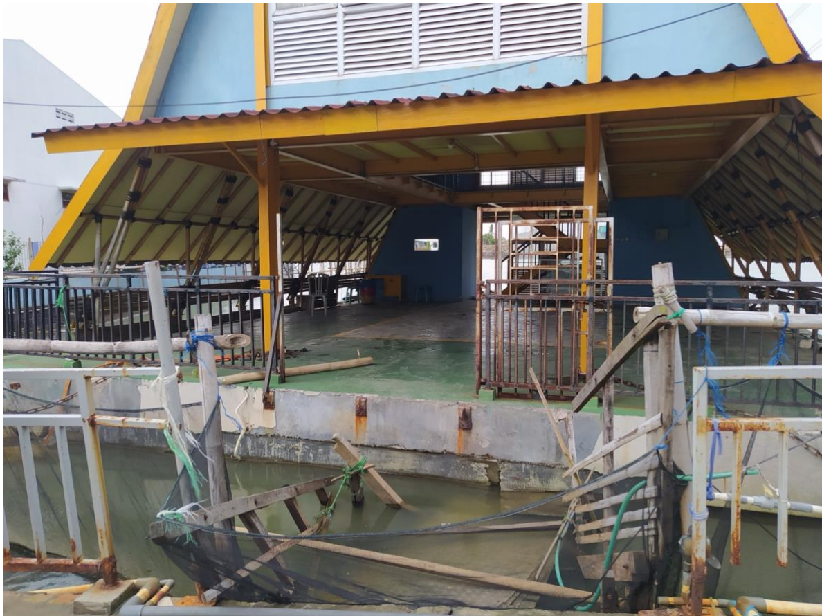
Figure 1 . Collapsed aspirations in slow ruin in February 2023 (Source: Authors' own).
